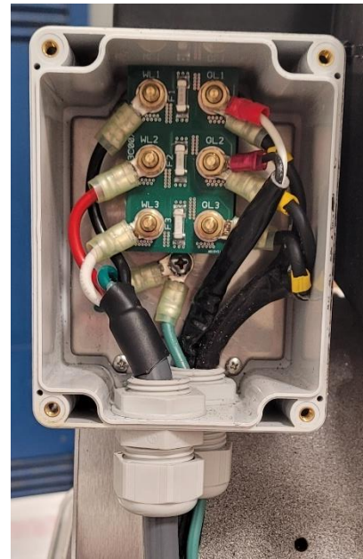
Figure 23 Fuse Board Connections
