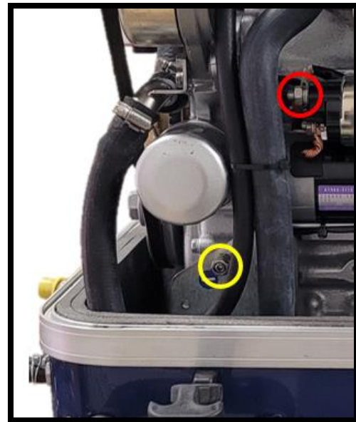
Figure 21: Starter Battery Cable Attachment Points
