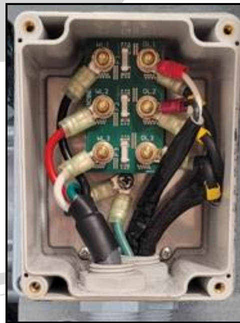
Figure 17: Fuse Board Connections
