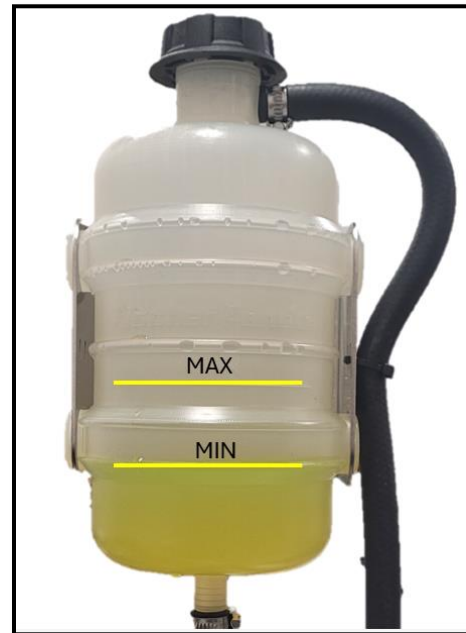
Figure 27: Coolant Expansion Tank
