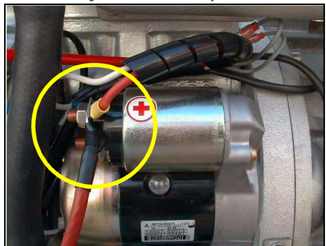
Fig. 5.8.1-1: Positive Battery Cable
