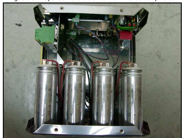
Fig. 5.9.3-2: Opened AC Control Box from Panda 30 upwards
