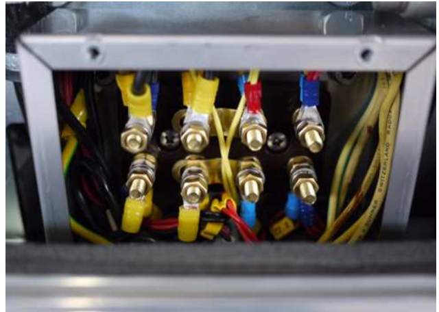
Fig. 4.3.6-6: Generator power terminal box
